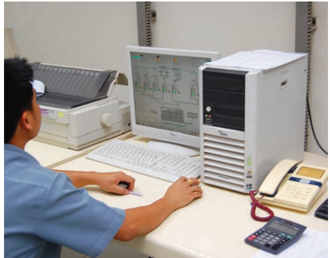
By optimizing the alarm system and implementing high performance HMIs, operators can detect disturbances as they emerge and intervene before an upset occurs.
